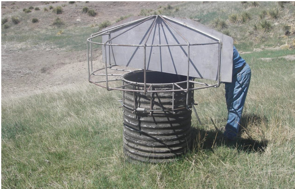
Example of an approved conical trash rack for vertical corrugated metal pipe risers.
