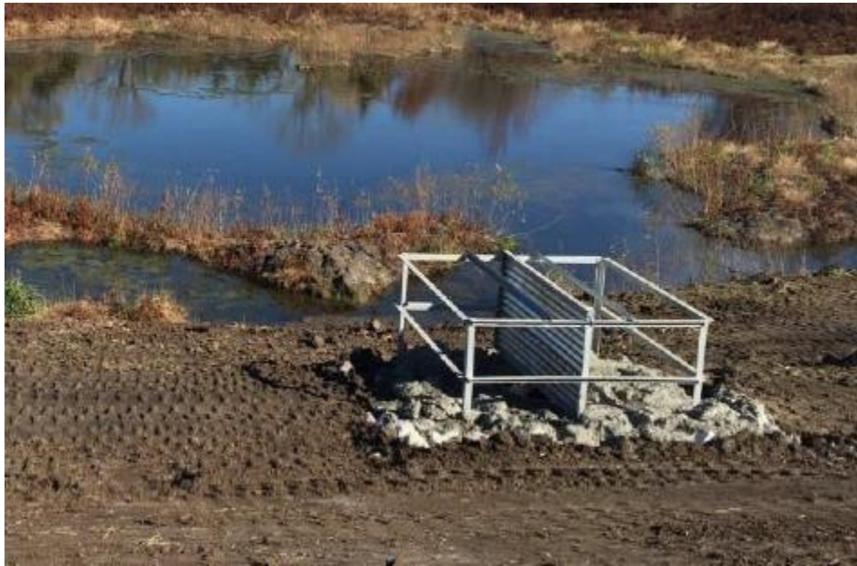
Another example of an approved trash rack for corrugated metal pipe risers.
