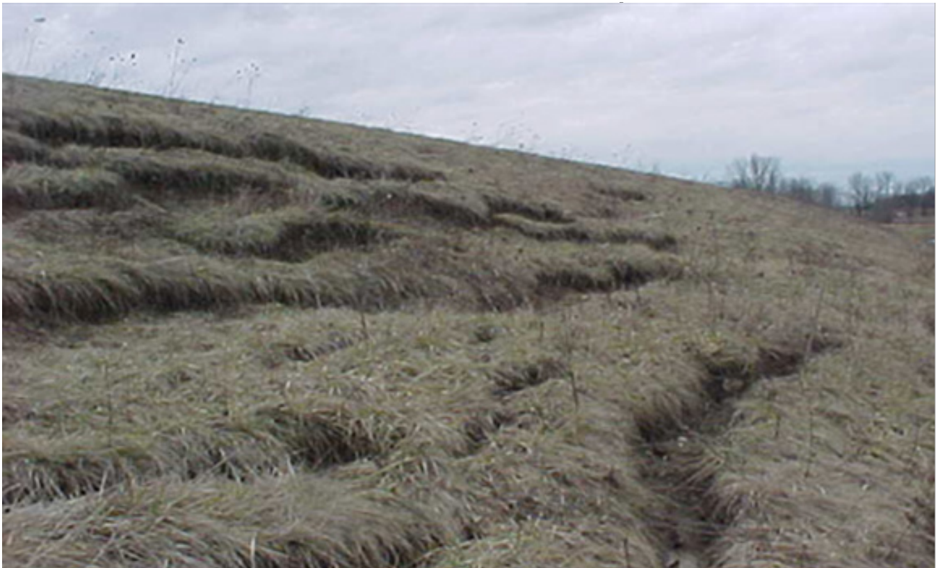
Figure 8: Slides on the Downstream Slope of an Embankment Dam
