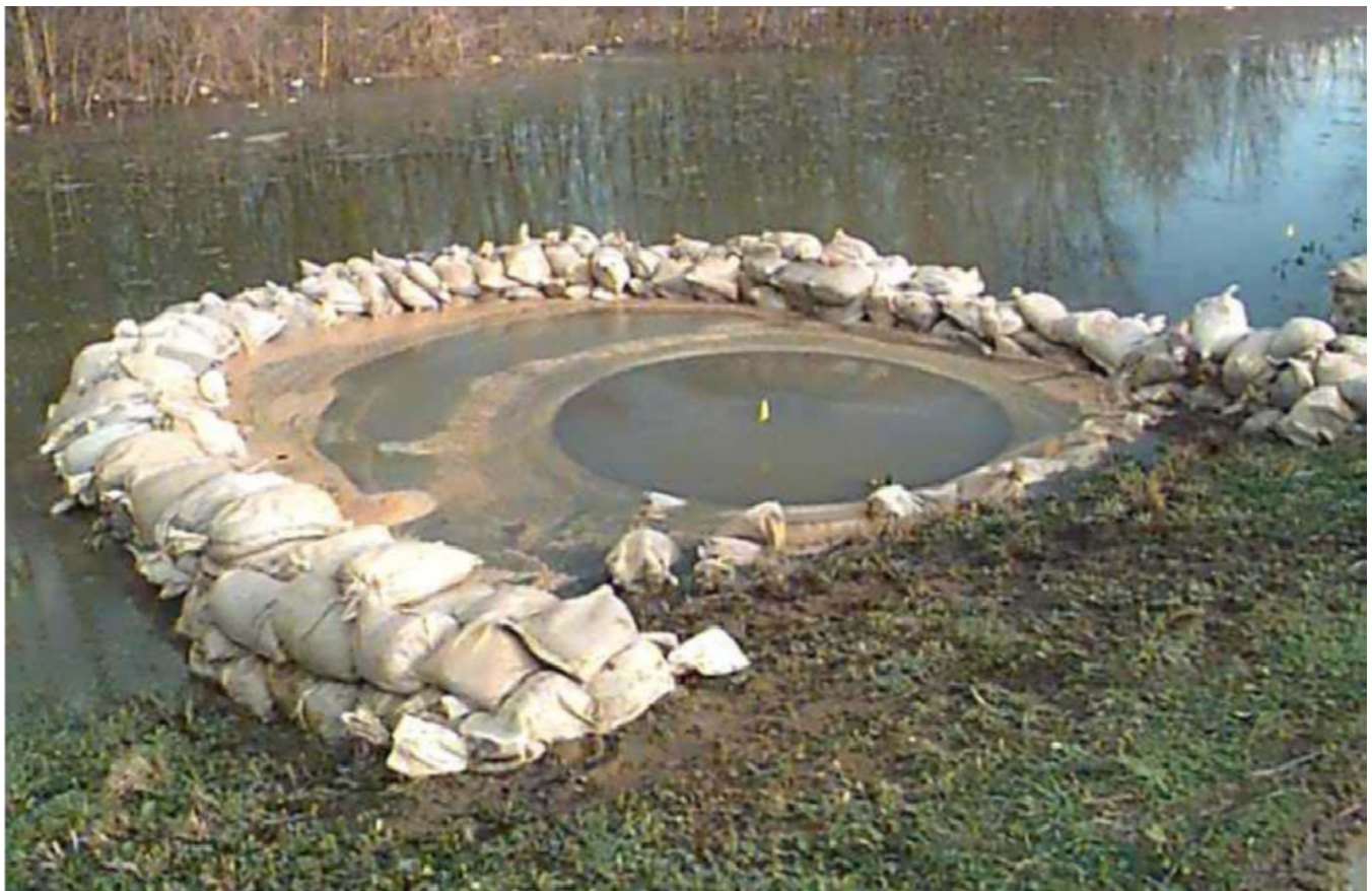
Figure 20: Sandbag Ring Levee around a Boil at the Downstream Toe of an Embankment Dam
