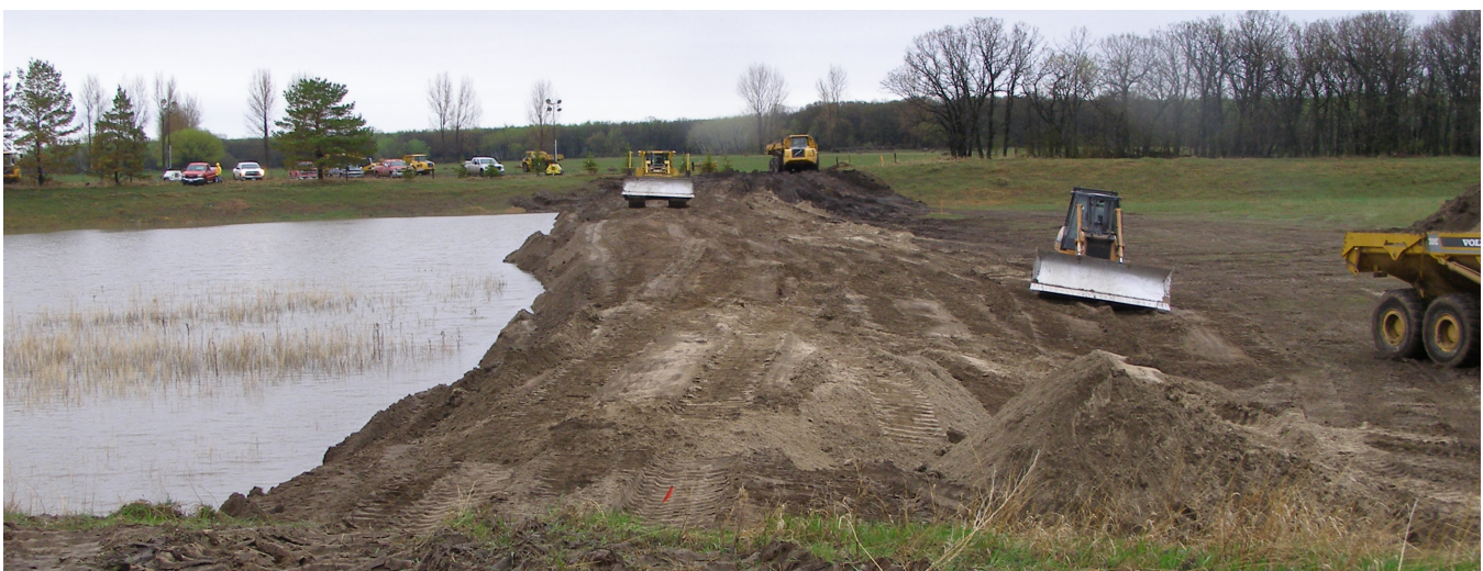
Figure 29: Construction of Temporary Fuse Plug across the Auxiliary Spillway Crest of Renwick Dam
