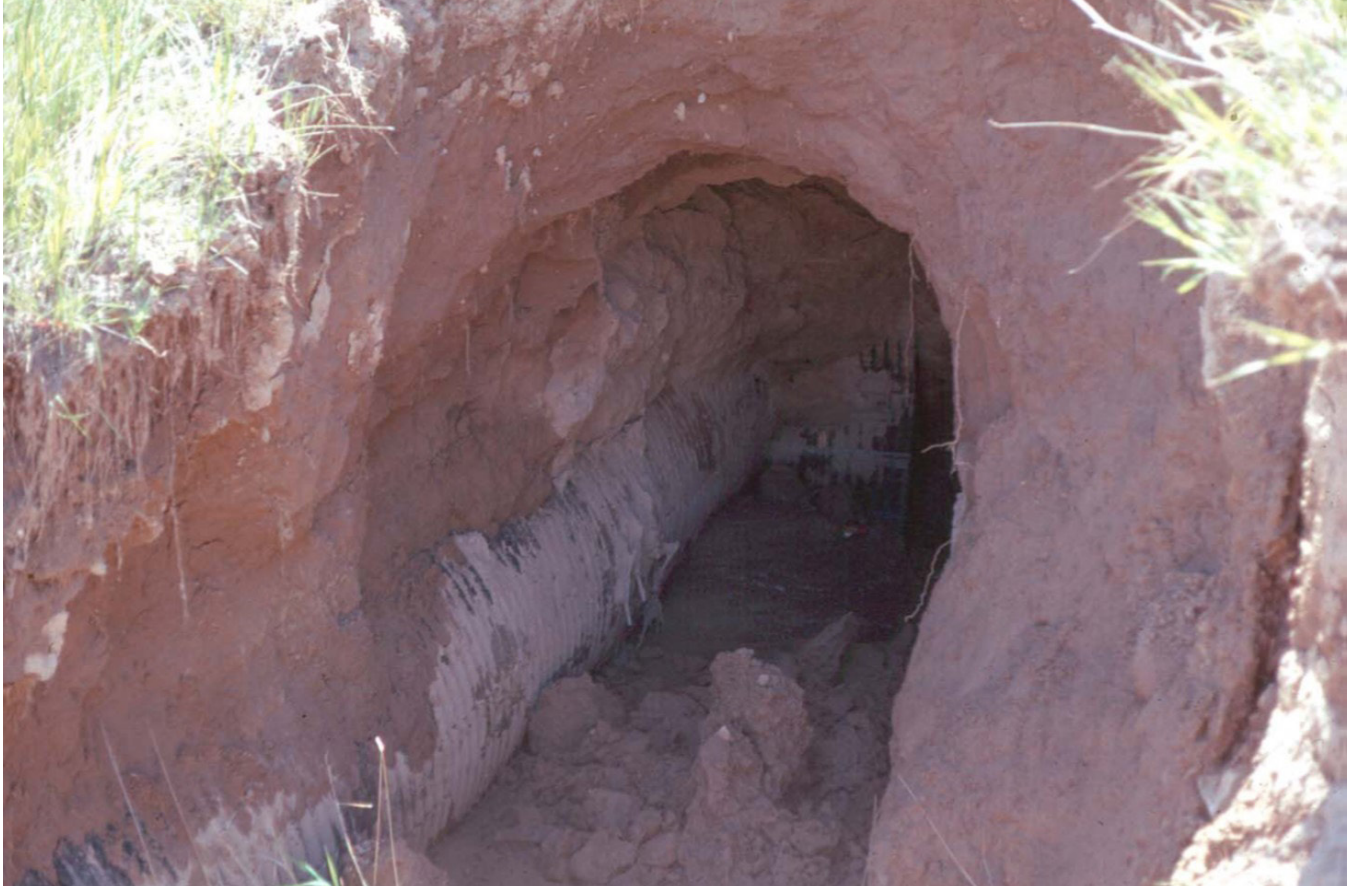
Figure 6: Photo of Internal Erosion Failure along an Outlet Conduit
