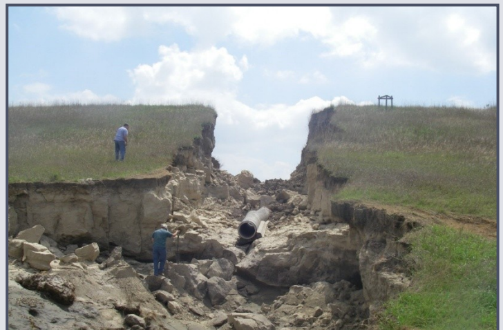
A transverse crack is believed to be the cause of this dam failure in Hitchcock County. Poorly compacted soil in the dam or in the foundation is the most common cause of transverse cracking.
