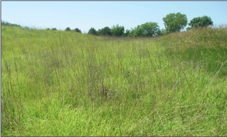
A well-maintained vegetated earthen spillway has a healthy, dense grass cover (no crops, vehicle ruts, or cattle paths) and smooth slopes (no abrupt transitions). Earthen spillways also must be kept free of obstructions that can collect debris and cause flow turbulence such as trees, fence lines, hay bales, and farm equipment.
