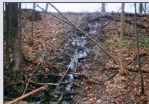
Seepage through dam damaged by tree roots. Trees should not be allowed to grow on dams. (Photo: ASDSO)
