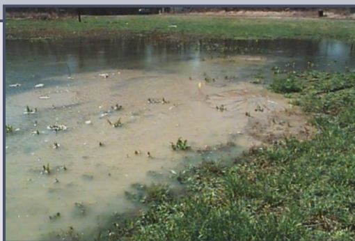
Severe example of a boil and seepage with significant cloudy flow. Cloudy flow is a sign that erosion is occurring inside a dam (Photo source: FEMA)
