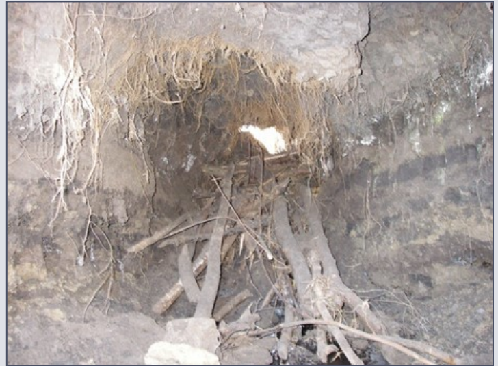
Looking inside a rodent hole that extended from upstream to downstream, entirely through a dam (Note daylight in center of photo).
