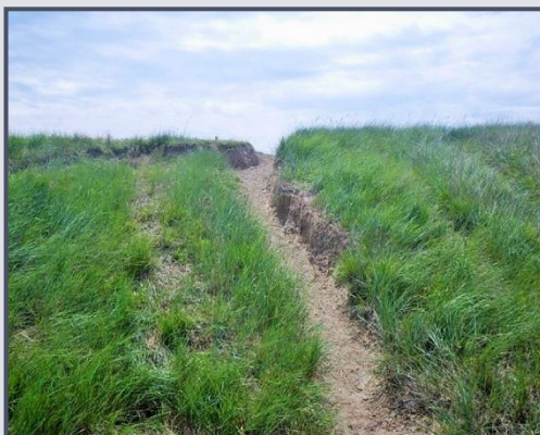
Dam embankment damaged by livestock.
