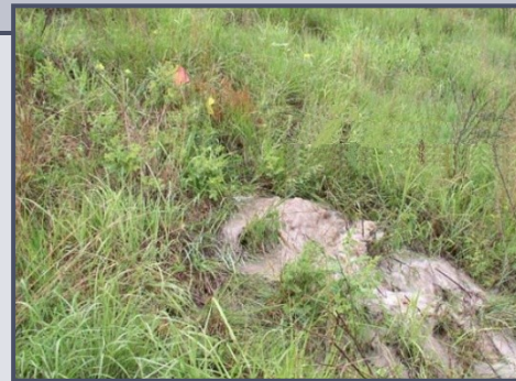
Cloudy seepage emerging from the downstream slope of dam in Frontier County, an indication that internal dam erosion was occurring. (Photo source: NRCS)
