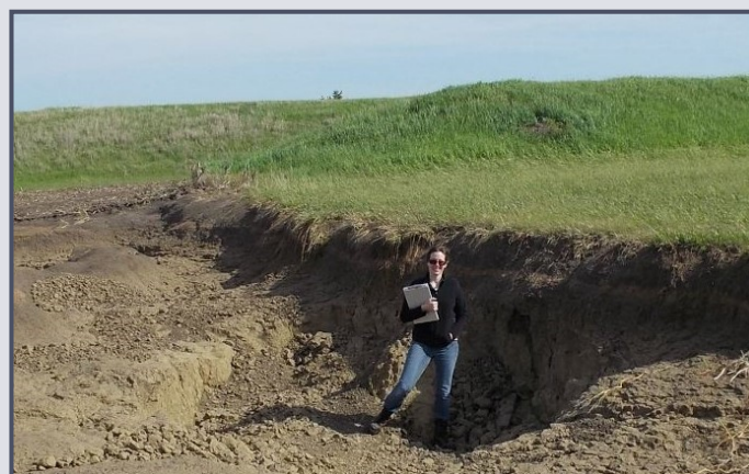
Erosion in auxiliary spillway where grass cover was removed and planted to crops.
