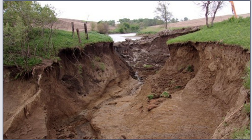
Failure of dam in Dixon County due to erosion in the vegetated earthen auxiliary spillway. A healthy, uniform grass cover is critical. One imperfection in a vegetated spillway, such as a small patch of dead grass, can be the starting point for erosion. Once erosion begins, the eroded area can quickly grow in size and breach the dam.
