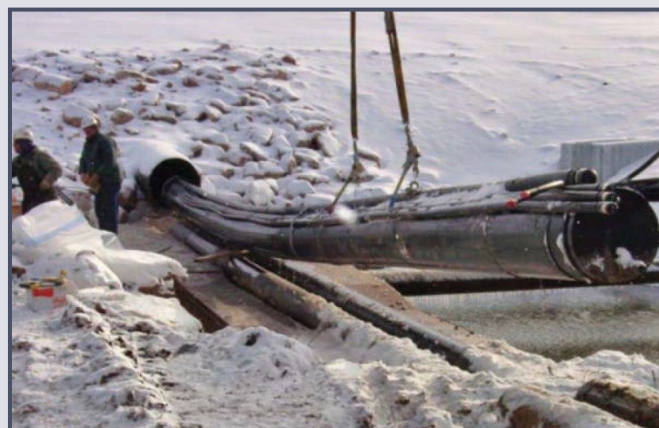
Rusty corrugated metal pipes can be sliplined with pressure-tight, solid-wall, HDPE pipe. Grout is injected into the space between the old and new pipes. (Photo source: FEMA)
