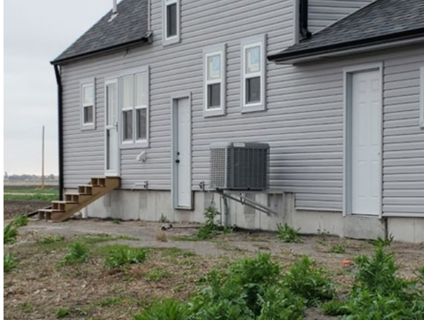
Figure 22: Air conditioner elevated to the same elevation as the lowest floor (first door on left side of image). (DWEE 2025)
