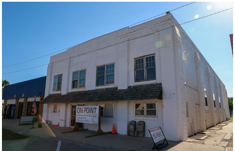
The Village of Kenesaw sits within the floodplain of the Thirty-Two Mile Creek watershed, and over 80% of the properties within the community—including the village's auditorium—are at risk of flooding. The Village will be floodproofing the building while also enhancing its functions. Image courtesy Jodi Randall, Village of Kenesaw.
